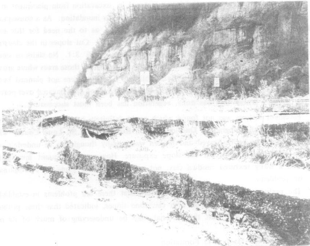
Figure 6. Abandoned Rte. 79 at Clarksville. (Roadway was relocated after green-type failures involving Maquoketa shale).
