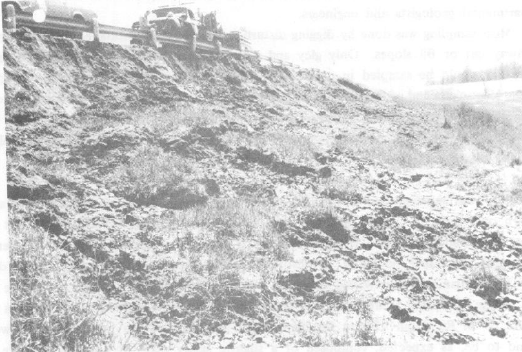
Figure 5. Progressive slope failure of fill built partially of gley on Rte. 63, Randolph County.
