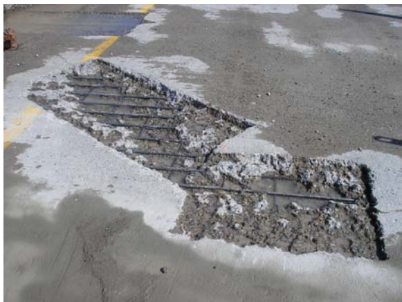
(5) Close Up Showing Exposed Rebar
