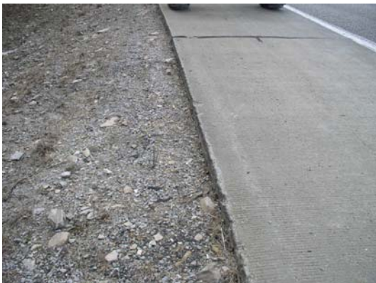
(11) Outside Shoulder Edge Prior to Edge Rut Repair
