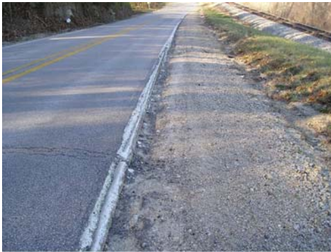
(1) Roadway Prior to Edge Rut Repair
