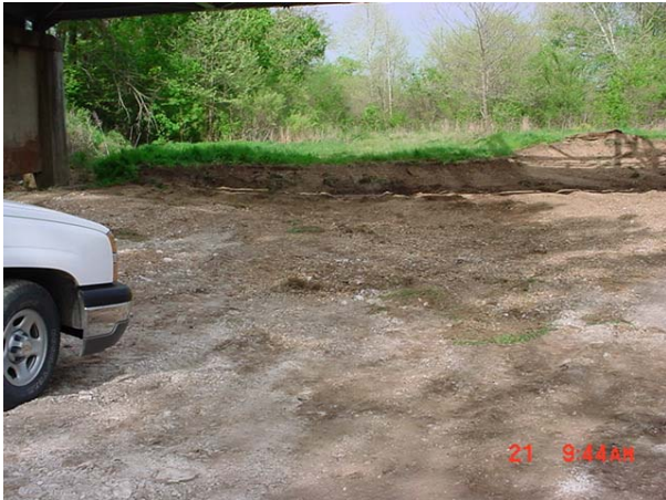
(9) Erosion under structure
