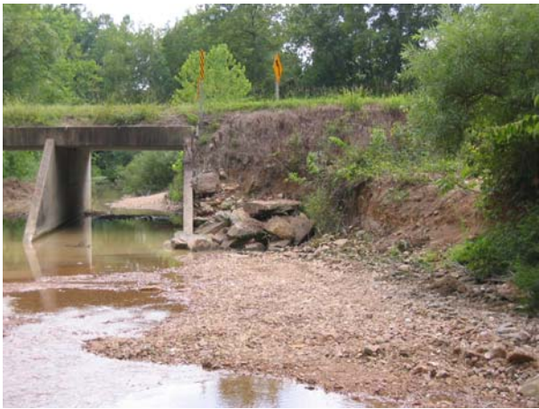
(1) Indian Creek -- Howell County Roadway Embankment Scour Upstream End
