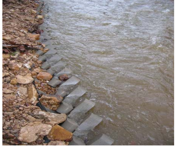
(8) Ajax Blocks Performing Under Full Flow Conditions
