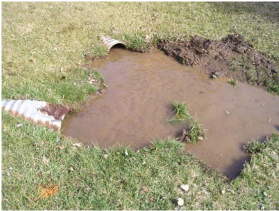
(1) Downstream Culvert Ditch (Silted In)
