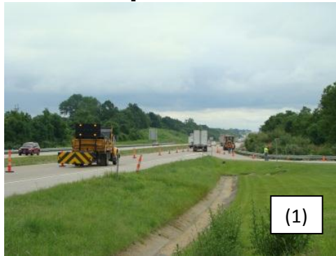
Picture 1 shows an acceptable exit ramp closure.
